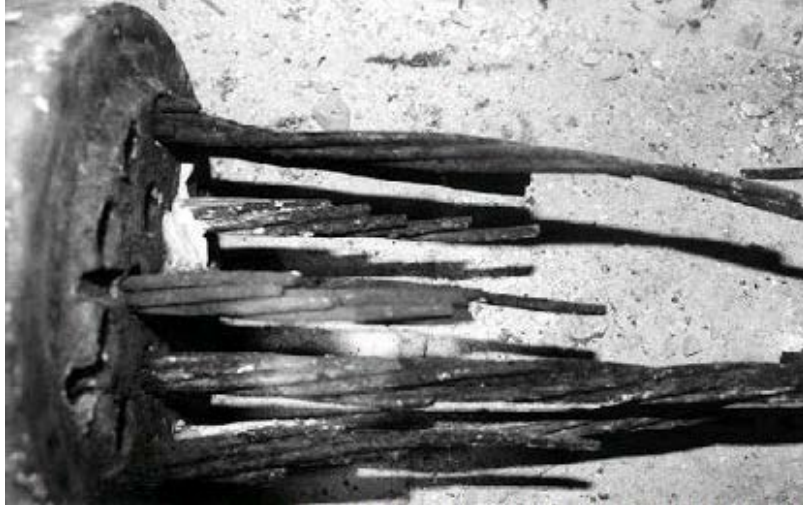
Figure 2.2. Strands corroded at anchor (Corven Engineering, 2002)
