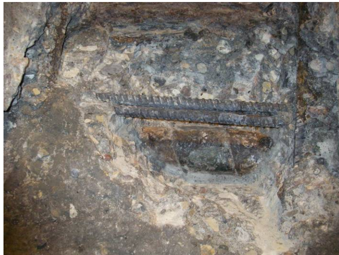
Figure 6.24. Shows tendon 16 with corroded duct
