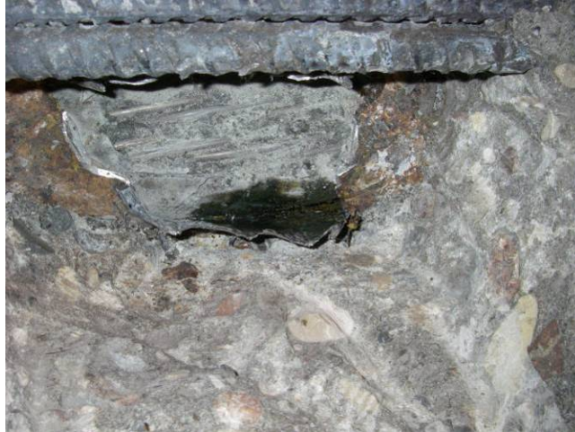
Figure 6.25. Opened tendon 16 with green corrosion product
