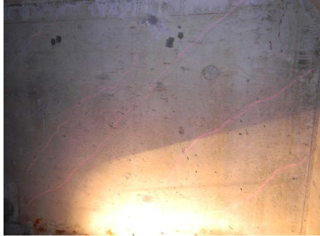
Figure 7.8. Diagonal cracking on interior of box girder
