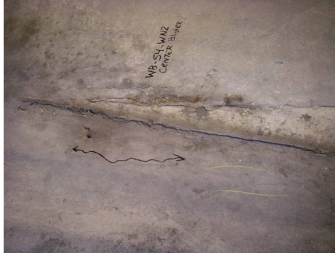
Figure 6.36. Cracking along anchorage blister in span 4
