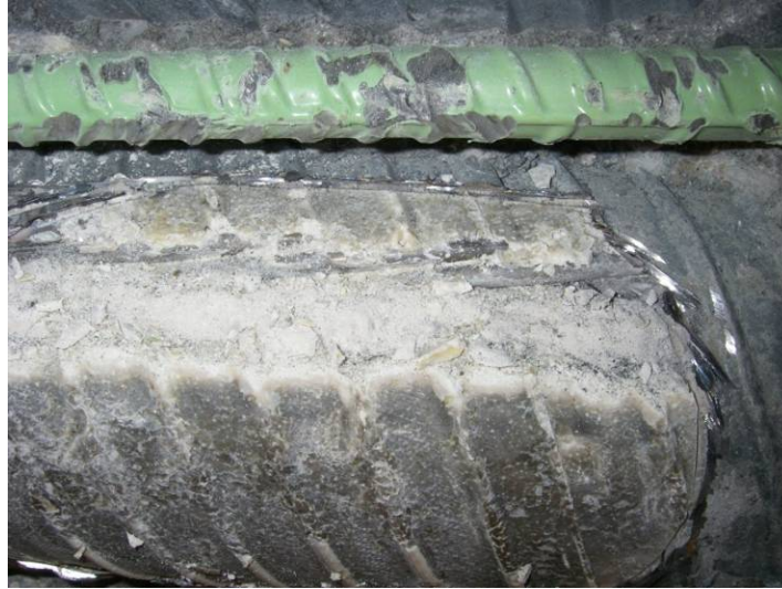
Figure 8.7. Bleed trail in tendon 2
