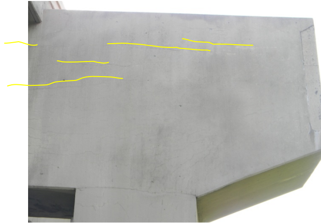
Figure 10.2. Cracking along straddle bent
