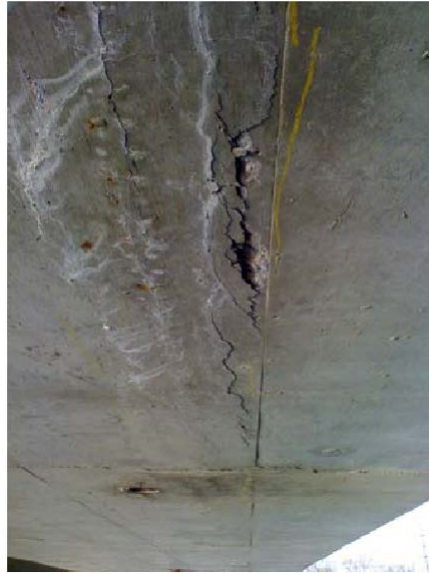
Figure 6.2. Bottom slab damage east to west view (Corven Engineering, 2010)
