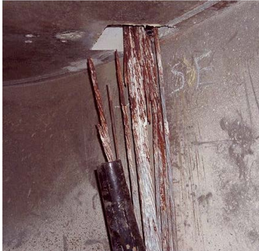
Figure 2.6. Corroded vertical tendons in Sunshine Skyway Bridge piers (Corven Engineering, 2002)
