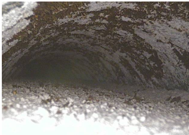
Figure 8.27. Borescope picture looking toward highpoint in tendon 3, 18 inches (45.7 centimeters) inside of the inspection hole
