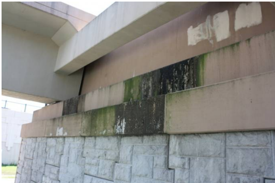
Figure 5.3. Discoloration of abutment
