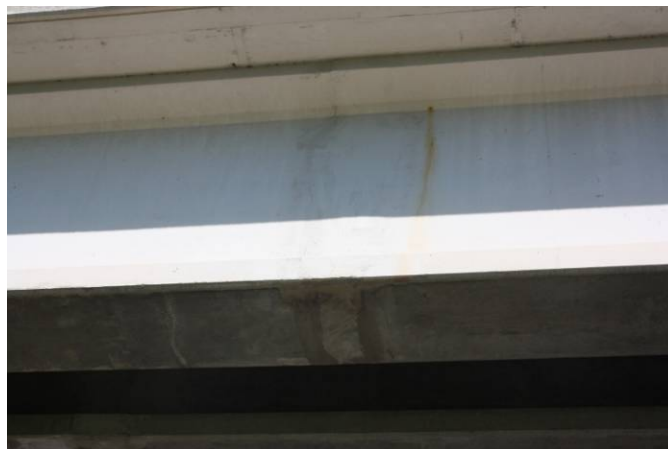
Figure 5.11. Moisture staining on exterior girder
