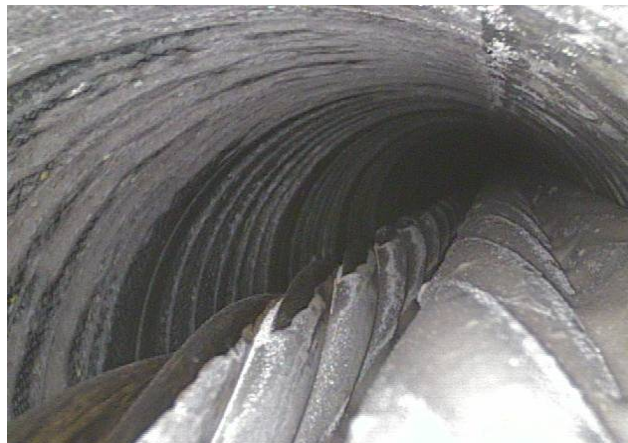
Figure 8.20. Borescope picture looking toward highpoint in tendon 3, 6 inches (15.2 centimeters) inside of the inspection hole
