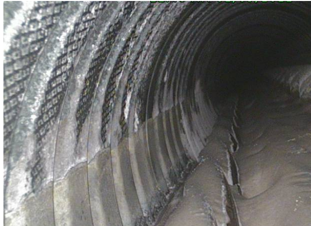
Figure 8.21. Boreoscope picture looking toward highpoint in tendon 3, 24 inches (61 centimeters) inside of the inspection hole
