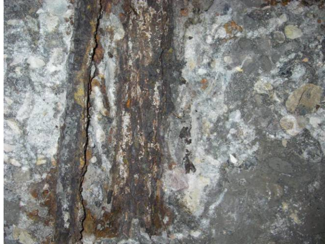
Figure 6.32. Corrosion on tendon B28
