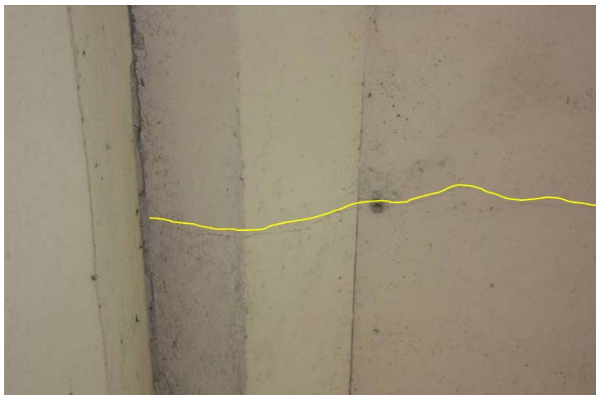
Figure 5.9. Cracking along box girder
