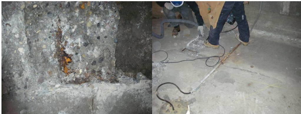
Figure 6.19. (Left) Corrosion product under spalling area at mid span
