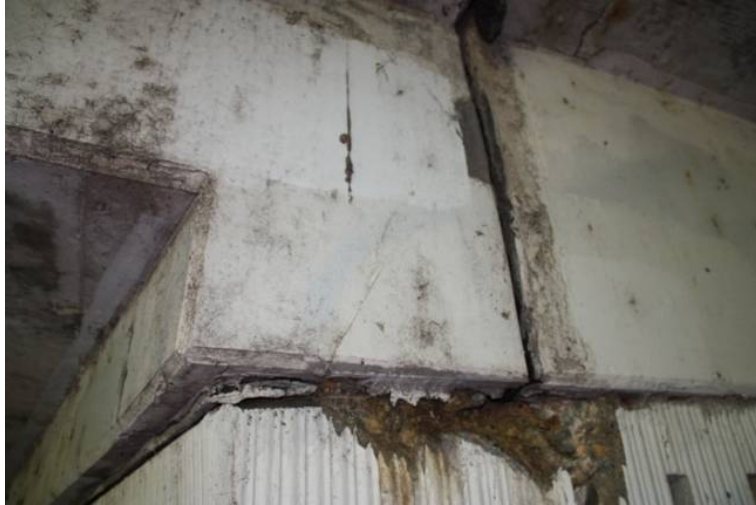
Figure 5.14. Spalling at abutment of bridge 27547
