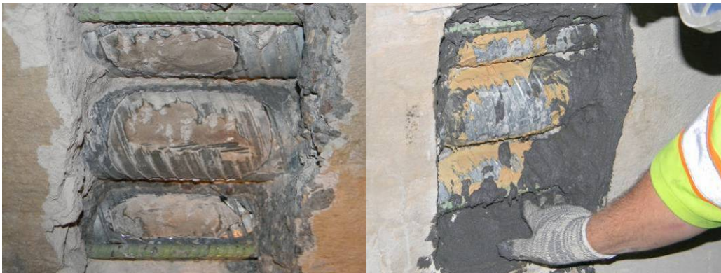
Figure 3.8. (Left) Exposed post-tensioning strand
