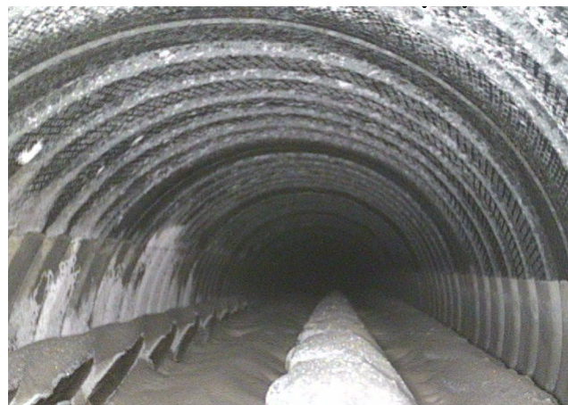
Figure 8.22. Boreoscope picture looking toward highpoint in tendon 3, 3.5 feet (1.07 meters) inside of the inspection hole
