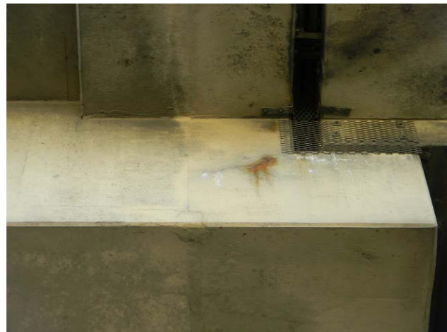
Figure 7.7. Cracking at connection of structural units
