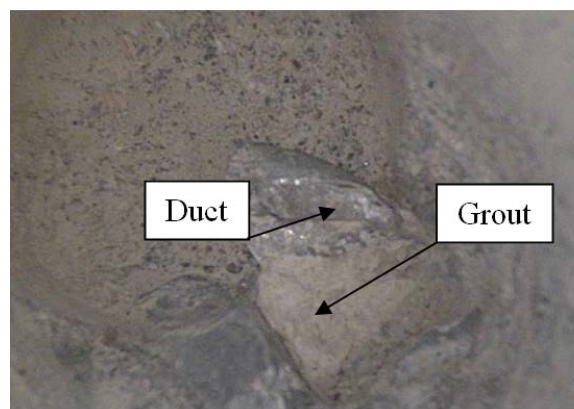
Figure 8.17. Borescope picture of drilled hole in girder 5 of span 3
