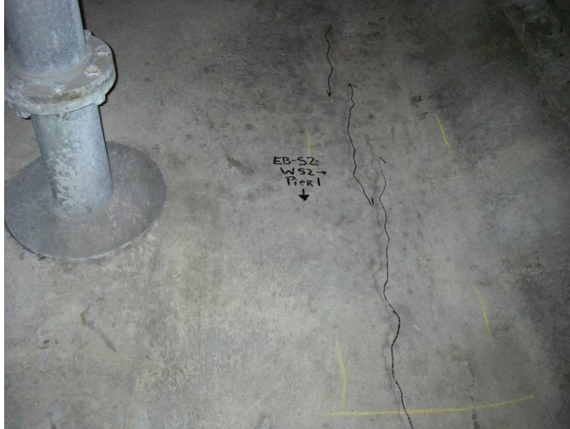
Figure 6.11. Cracking in span 2 eastbound structure
