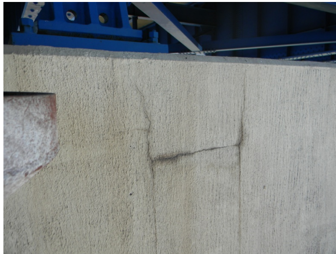
Figure 9.3. Vertical and horizontal cracking in pier
