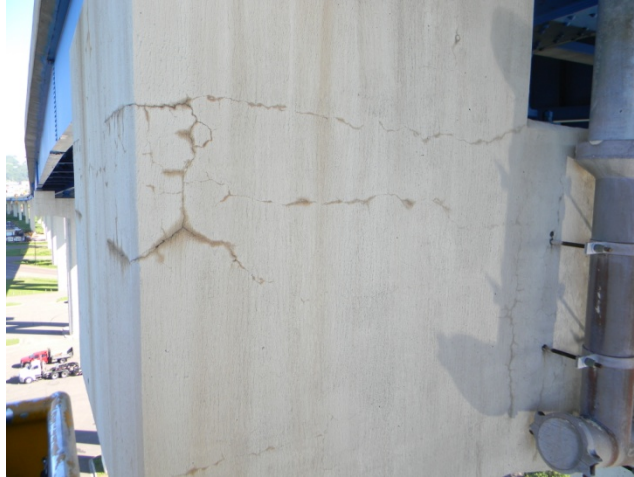
Figure 9.2. Cracking extending from anchorage on PT pier cap
