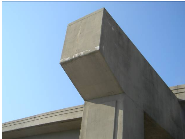
Figure 10.1. Pier with cracking and efflorescence
