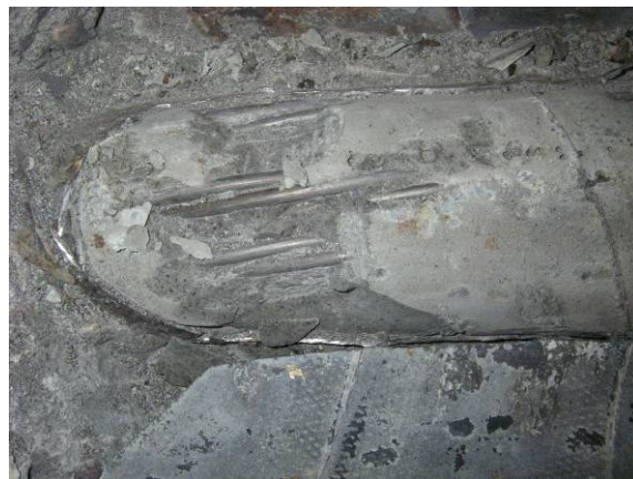
Figure 6.26. Tendon B15 with removed window exposing multiple strands
