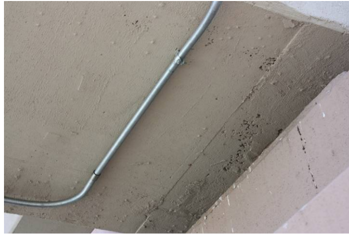
Figure 5.4. Honeycombing along bottom of box girder
