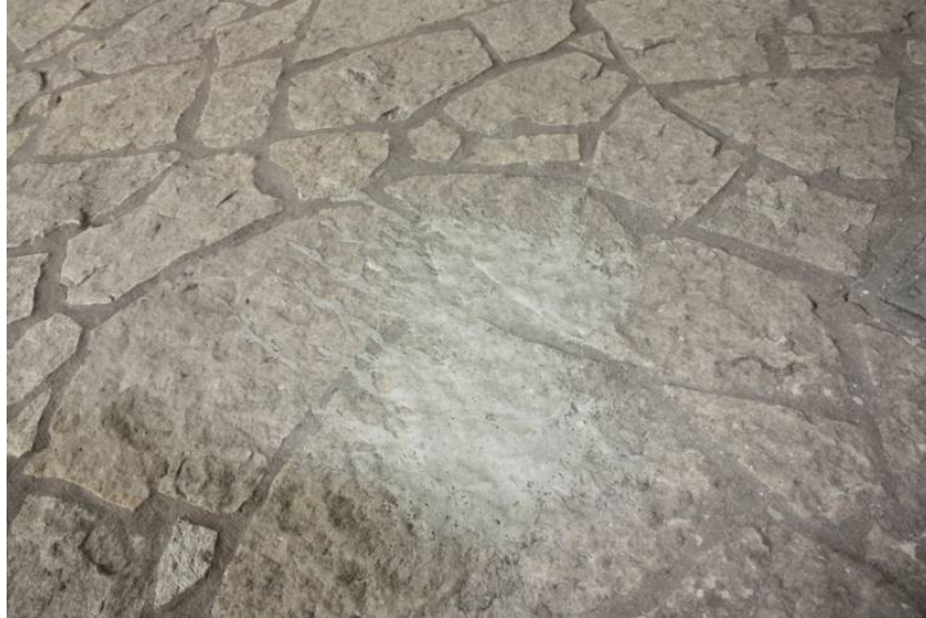
Figure 5.8. Grout splatter beneath access hatch
