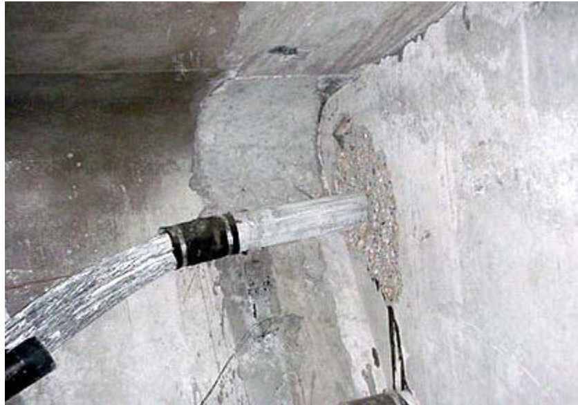
Figure 2.4. Tendon at expansion joint were failure occurred (Corven Engineering, 2002)
