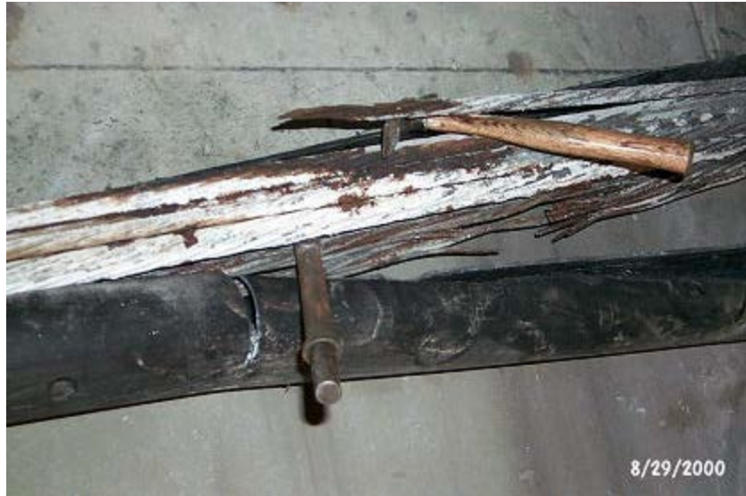
Figure 2.5. Corroded tendons at breached duct (Corven Engineering, 2002)
