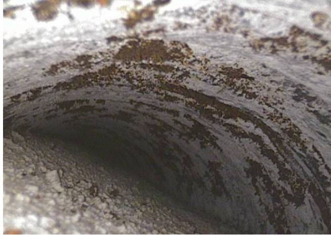
Figure 8.28. Boreoscope picture looking toward highpoint in tendon 3, 5.5 feet (1.68 meters) inside of the inspection hole
