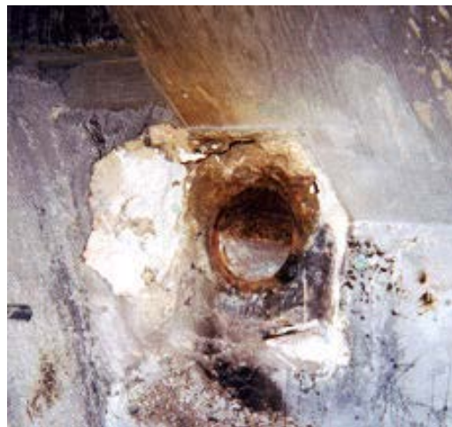
Figure 2.3. Water staining at expansion joint around anchor where tendon corroded (Corven Engineering, 2002)
