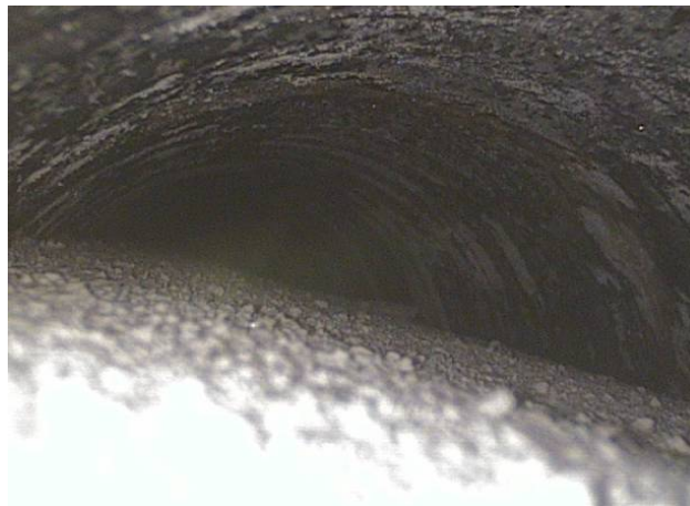
Figure 8.29. Boreoscope picture looking toward low point in tendon 3, 46 inches (116.8 centimeters) inside of the inspection hole
