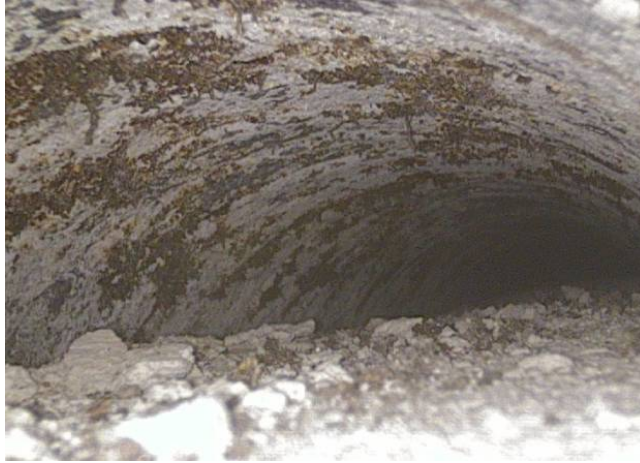
Figure 8.26. Borescope picture looking toward highpoint in tendon 3, 6 inches (15.2 centimeters) inside of the inspection hole
