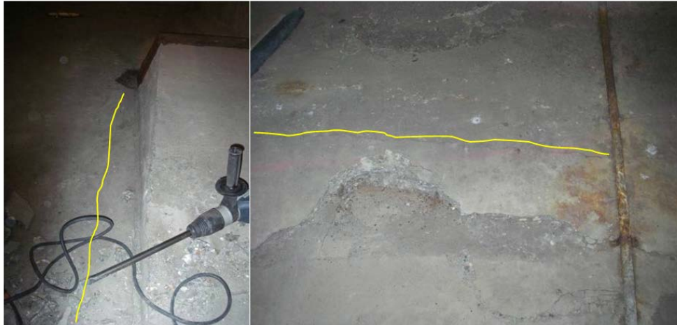
Figure 6.27. (Left) Crack along anchorage of tendon B28/B24
