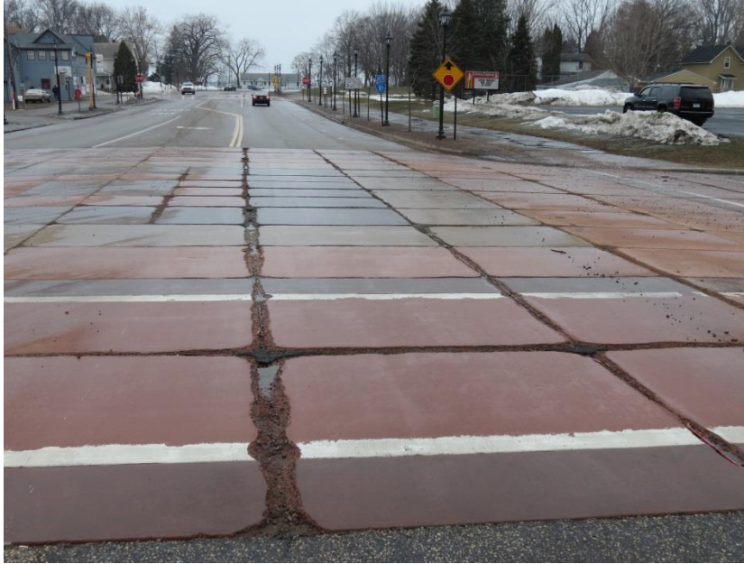
Deteriorating crosswalk in Centerville, MN
