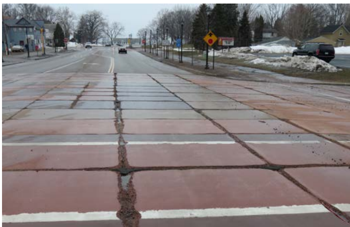
The City of Centerville plans to tear up its colored concrete due to early joint deterioration.
