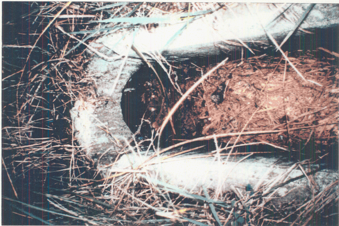
Figure 3. Photo of typical I-90 (Austin, MN) drain outlet, 1994.
