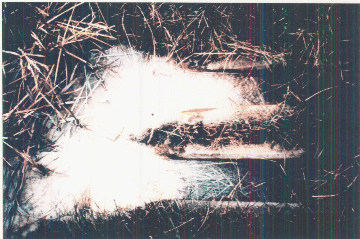
Figure 4. Precipitate around I-90 (Austin, MN) drain headwall.
