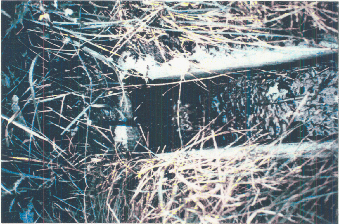
Figure 1. Photo of typical I-90 (Austin, MN) drain outlet, 1987.
