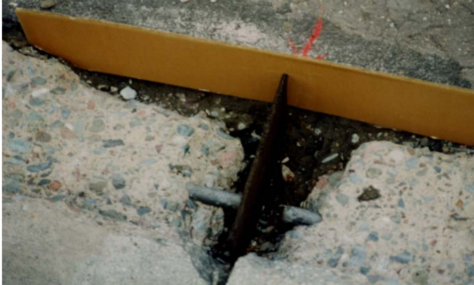
Figure 4.6 Common view of edge deterioration going to bottom of pavement.
