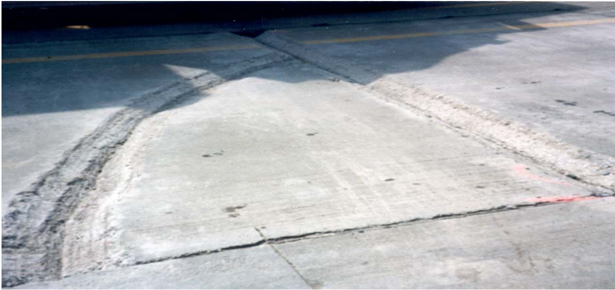
Figure 4.1 View of partial depth repairs after milling operations, both a joint and a crack.
